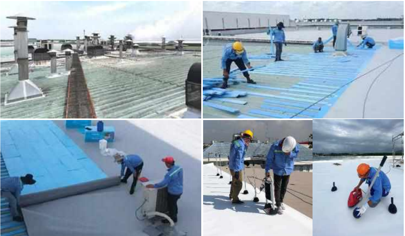
Install Roofcare UltraPly TPO membrane system/ Thi công hệ Roofcare UltraPly TPO
